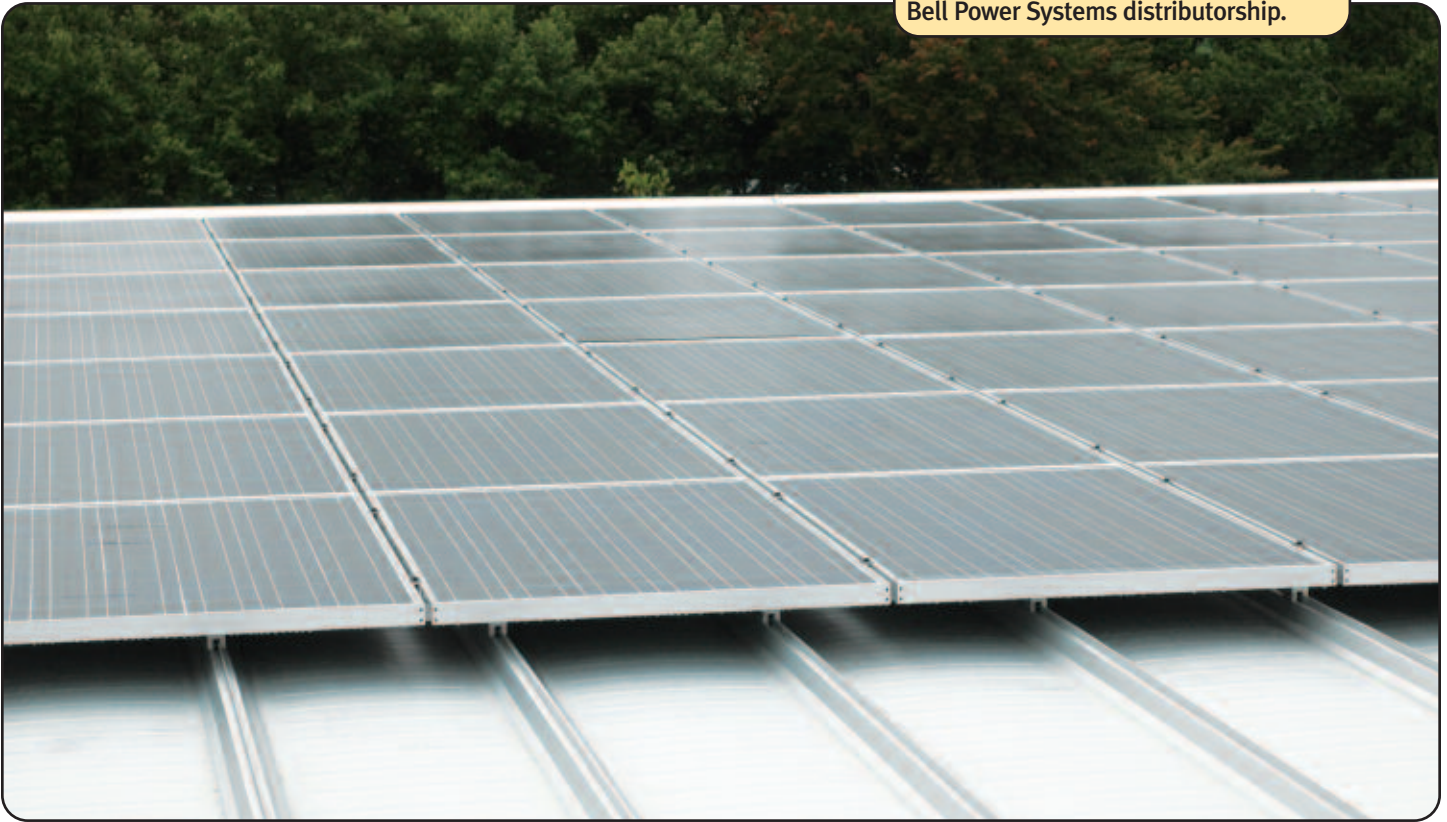
Solar Array panels grace the roof of the Bell Power Systems distributorship.
